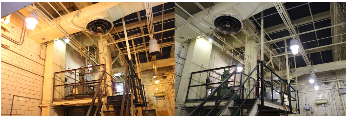
Before: 250W High Pressure Sodium Lamps
